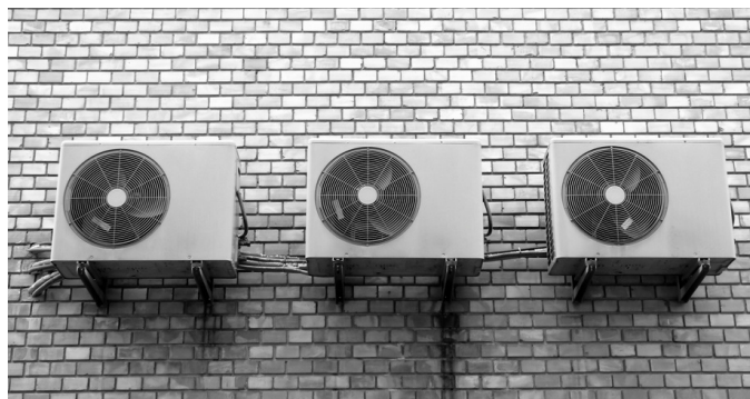
Air Conditioning, Air Scrubber
